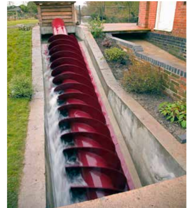
Left: LAPD Architects utilised an Archimedes screw as part of their strategy to generate energy from the waterway on this site
